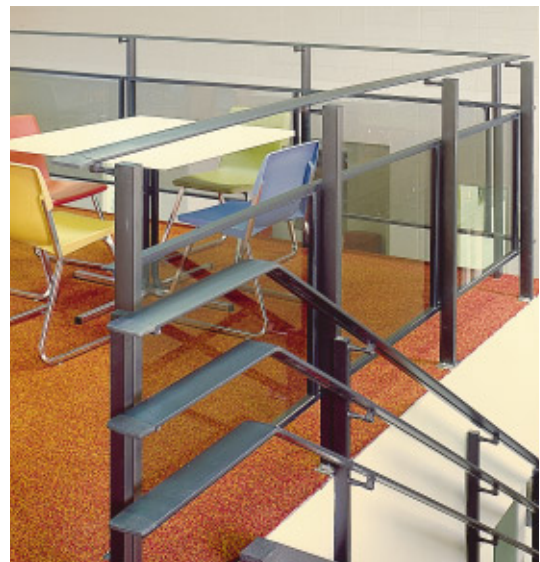
AMERICUS HIGH SCHOOL Americus, Georgia Arch.: James W. Buckley & Assoc. Fabr.: Architectural Manufacturing Company of America
